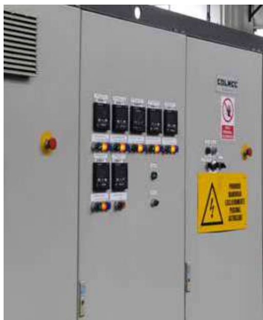
Switch cabinets for line control
